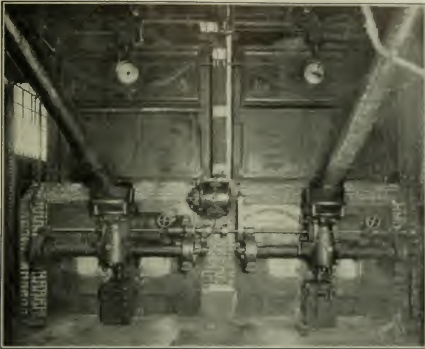
FIG. 3 ELLIOTT MECHANICAL STOKERS AT THE RIDGWAY DYNAMO AND ENGINE COMPANY'S PLANT
